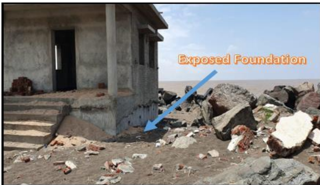
Foundation exposed due to erosion at Nani Danti- Moti Danti
