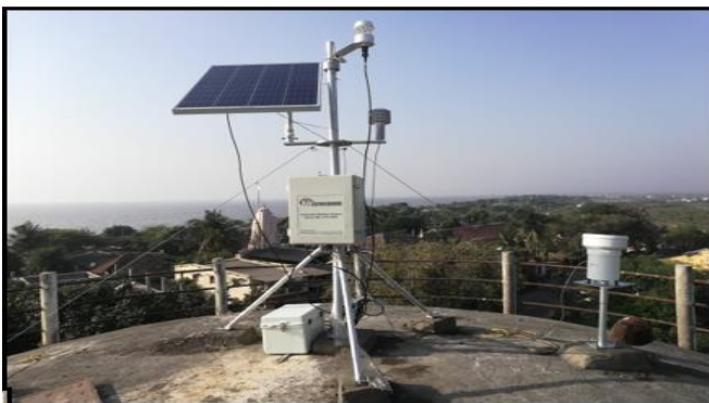
Automatic Weather Station (AWS) installed at Nani Danti- Moti Danti
